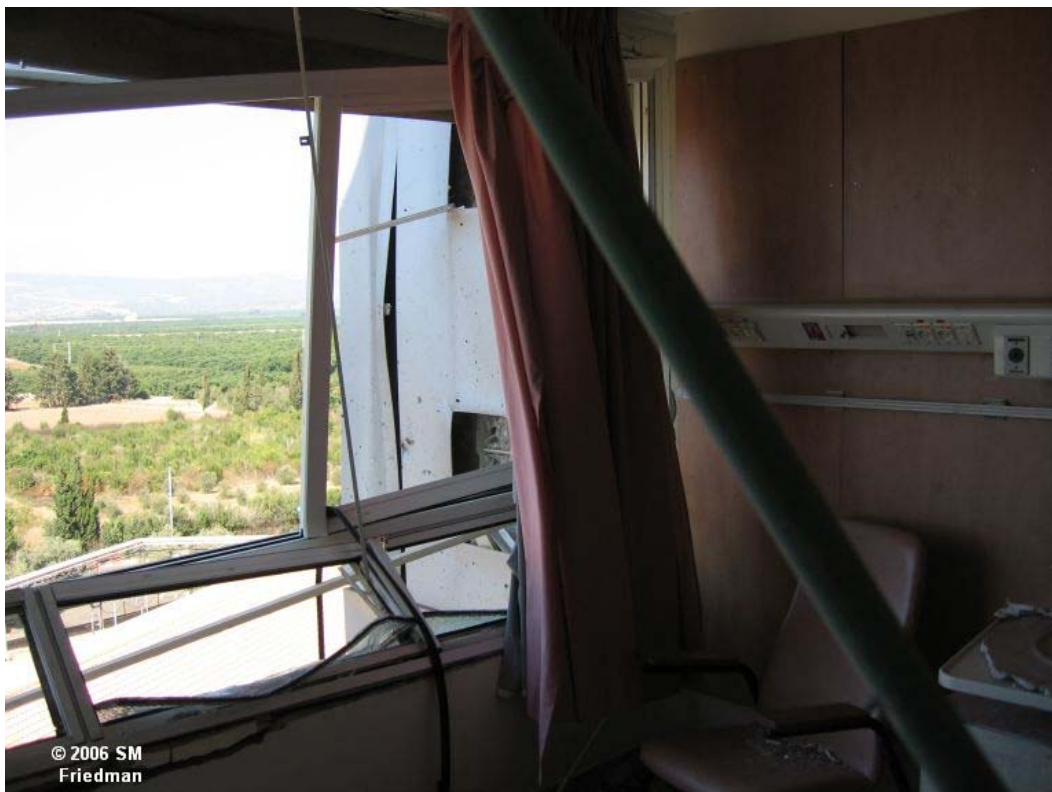
Katyusha missile damage on hospital room, Western Galilee Hospital, Nahariya, Israel.
