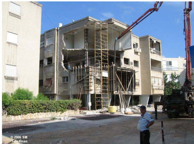
Katyusha missile damage on residential building , Bat Galim, outside Haifa, Israel.
