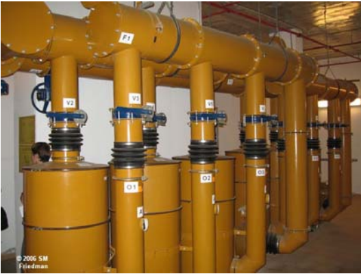
Closed Air Filtration System for protection against biohazard.
